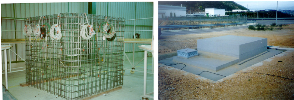
Fig. 9. Reinforcement of the pilot container with corrosion sensors and its aspect once buried. There is a main hole to have access to the chamber where the corrosion-data logger is placed besides the container.
